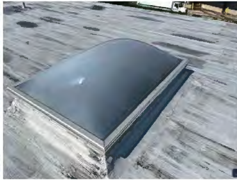
Warehouse Roof Southwest- Repair/replace
