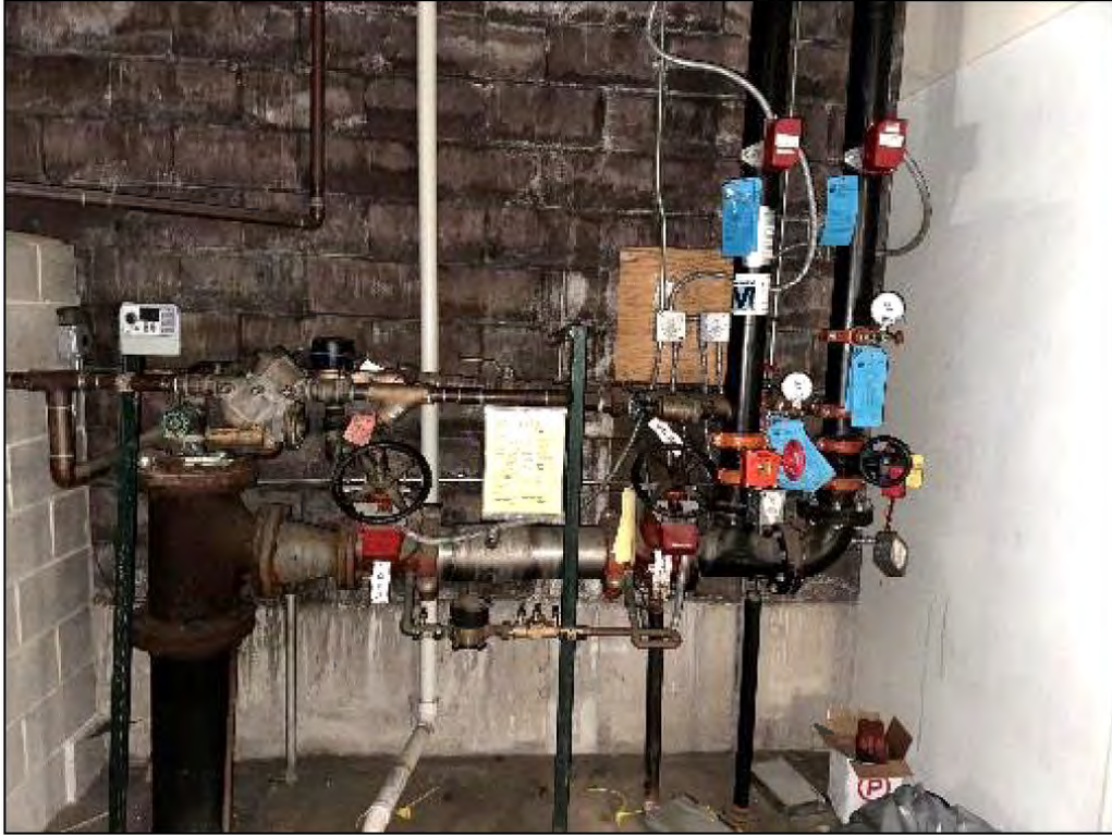
Sprinkler System and Controls
