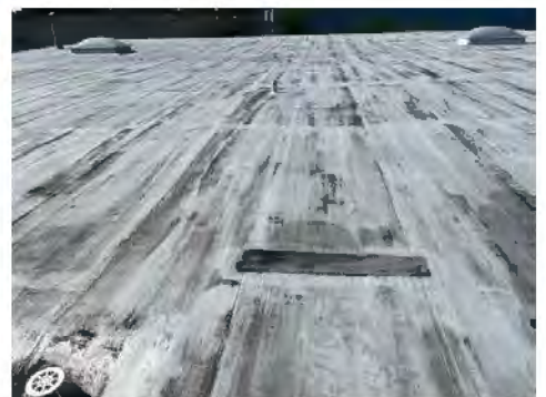
Maintenance is needed
