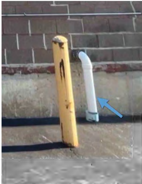
South- Regular maintenance is needed
