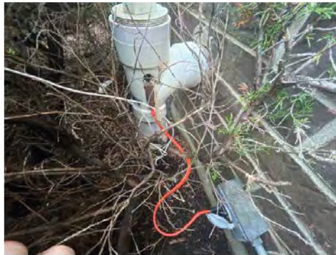
West- Regular maintenance is needed
