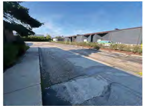
Maintenance is needed
