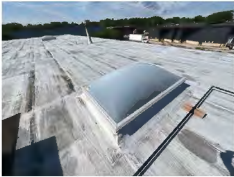
Warehouse Roof West- Repair/replace
