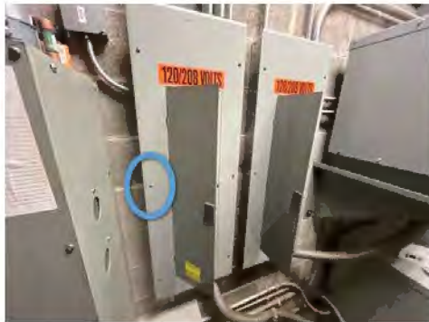
Main Office Electrical Room- Replace
