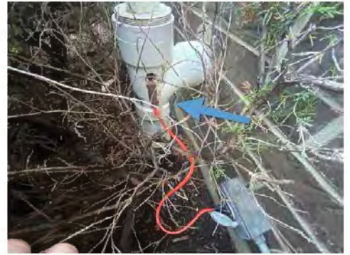
Evaluate & Repair As Needed
