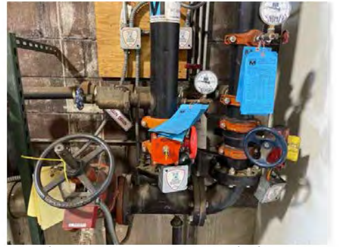
Regular maintenance is needed
